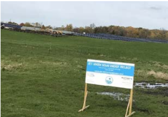
Watertown, Minnesota, USA Solar Garden
